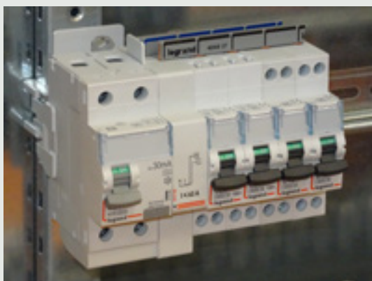
It is possible to mix screw connection and automatic terminal connection MCBs on the same row
