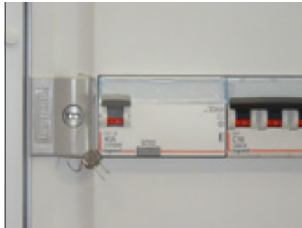
Sealing the faceplate, in locked position
