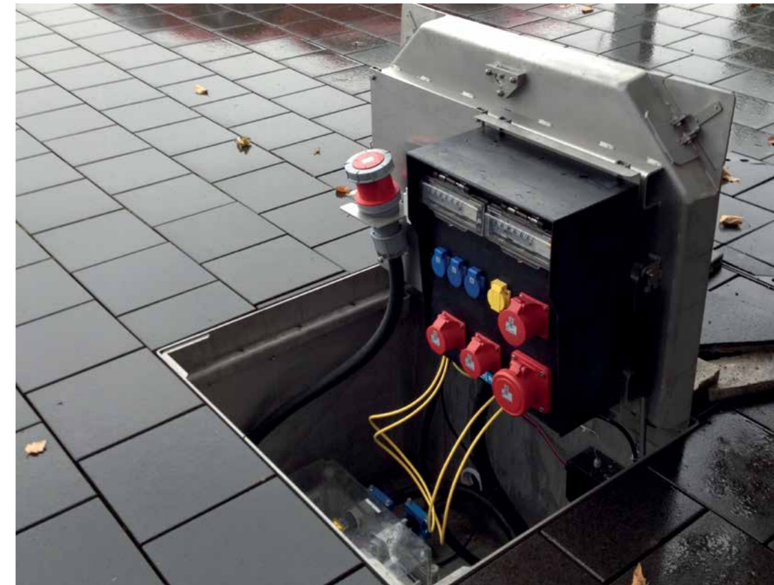
Retractable supply post with hatch cover
